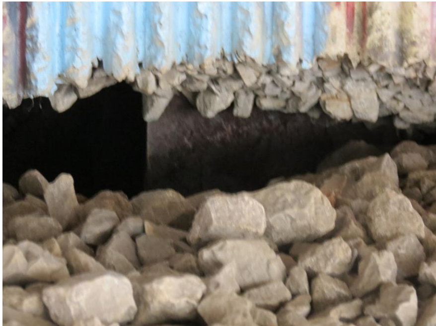
EXP. PILE W/ CORROSION AT ABUT. #2
