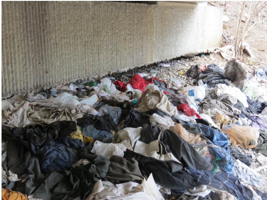
SETTLEMENT AT ABUTMENT #1
