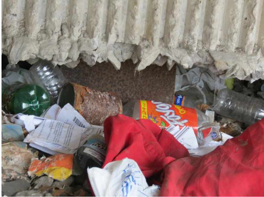
EXP. PILE W/ PITTING AT ABUT. #1
