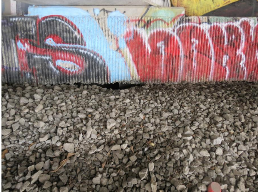
SETTLEMENT AT ABUTMENT #2
